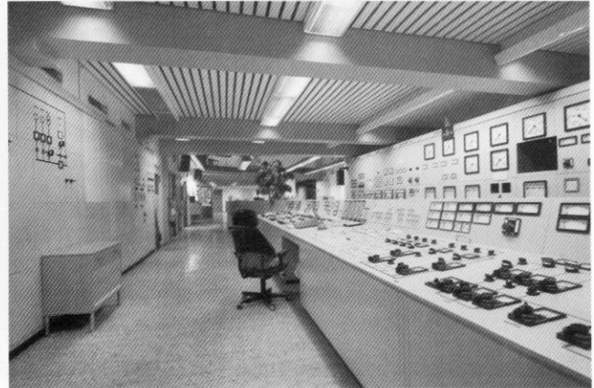
The newer control room for generators 3 & 4
